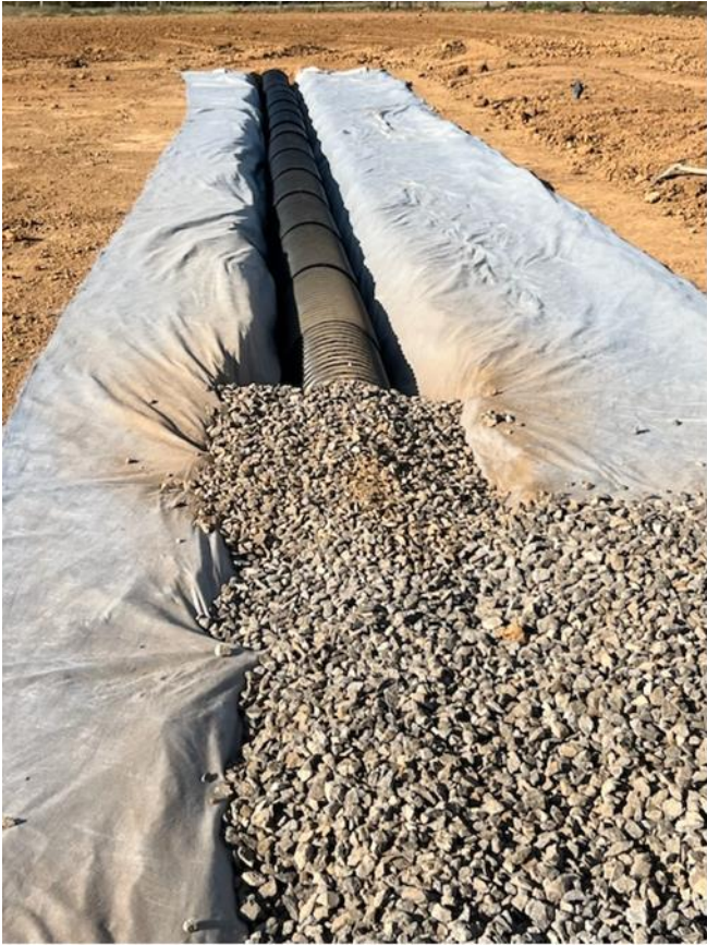
Image 17: Backfilling of Wick Trenches, with Geotextile fabric lining the trench before backfilling with suitable sized rock and arch drain.
