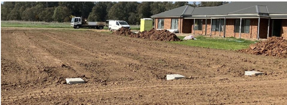
Image 15: Completed work – top of each trench is domed above natural ground so that surface water/rain does not sit on top of the trenches.
